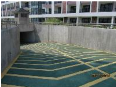
Exhibit: No shock&slip slope road
